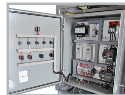
user friendly PLC controls with HMI interface in a UL certified panel
